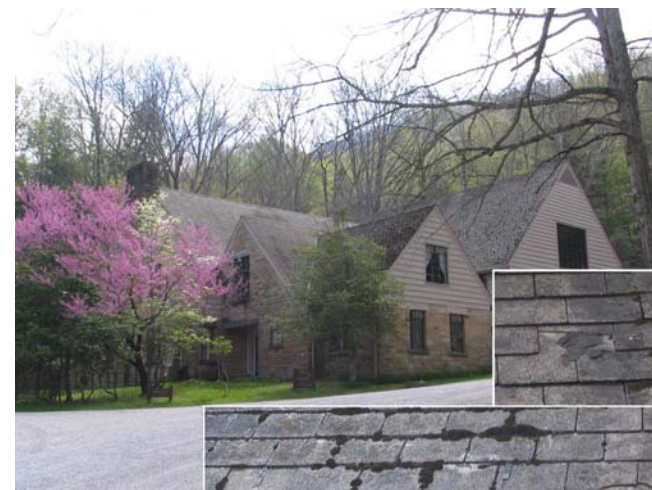
Insets show damaged shingles on Laurel House roof
