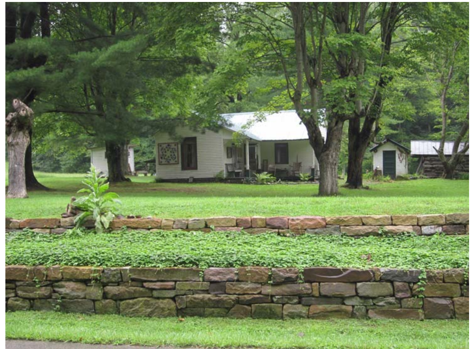
After taking a dry stone workshop at the Settlement School, artist Jeff Chapman-Crane built this 120-foot, terraced retaining wall in front of Valley of the Winds Art Gallery on State Route 806 in Eolia, Kentucky.
